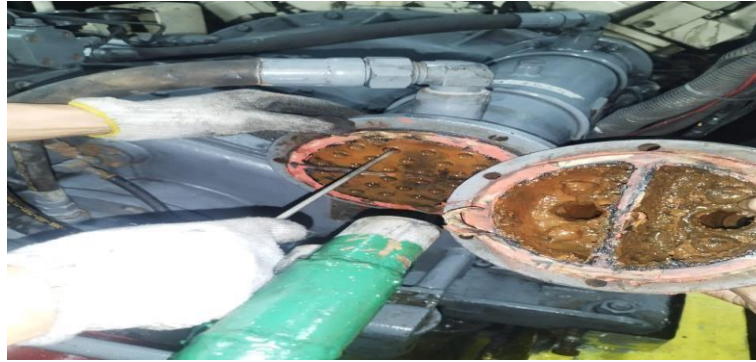
Figure 6 Cooler Gear Box Source: Documentation 2024
