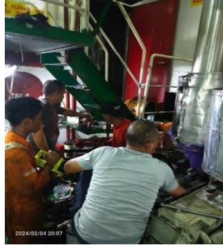
Figure 10. Checking the temperature of the primary engine cooler Source: Documentation 2024
