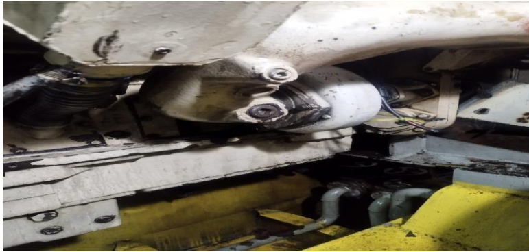
Figure 4 Fresh water pump. rce: Documentation 2024
